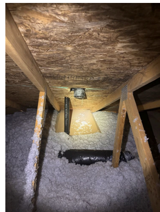
Hallway bathroom duct
