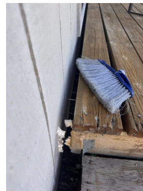
Deck improperly attached to house.
